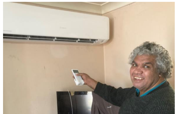
Split system units installed to 34 Cowra LALC properties
